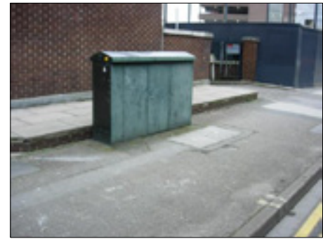
PHOTOGRAPH 6 EXISTING VIRGIN MEDIA CHAMBER AND CABINET IN GERARD STREET ADJACENT JUNCTION WITH GREYFRIARS ROAD
