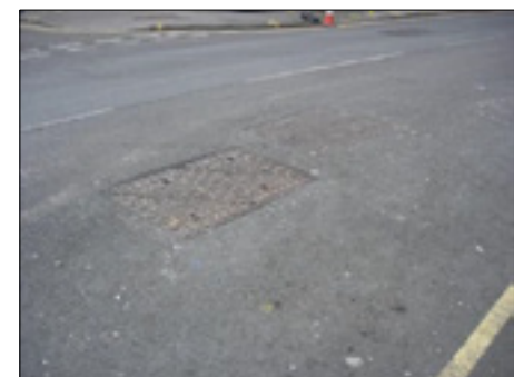
PHOTOGRAPH 3 EXISTING VODAFONE AND CITY FIBRE CHAMBERS IN GREYFRIARS ROAD OPPOSITE VACHEL ROAD
