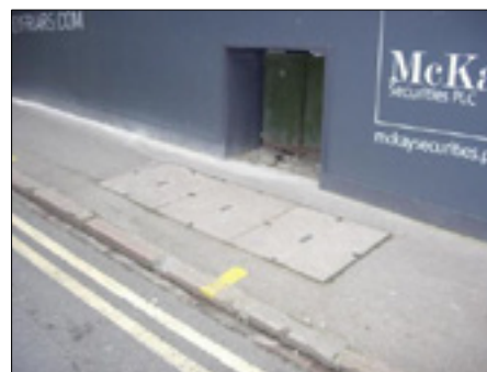
PHOTOGRAPH 2 EXISTING BT CHAMBER AND CABINET OUTSIDE OF BUILDING IN FOOTWAY ON GREYFRIARS ROAD
